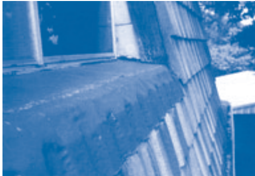
Weathered asbestos roofing
